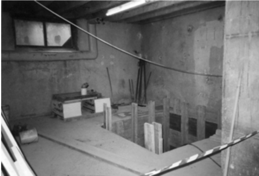
July 2000: Preparation of the installation of the Tecnai F20: Construction work in the cellar of the building Steyrergasse 17
