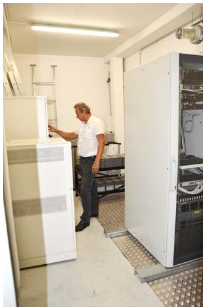
The new server room with the new uninterruptible power supply system.
